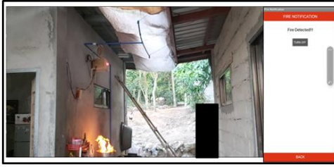
Figure 19. Flame Sensor and Automatic Water Sprinkler
