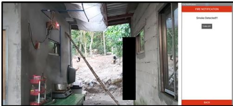
Figure 20. Smoke Sensor and Automatic Water Sprinkler
