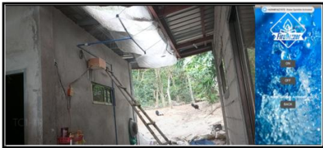
Figure 17. Manual Water Sprinkler and Switch (video reference:
